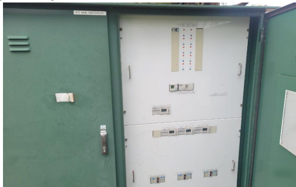
Figure 9-4: Main switch board
