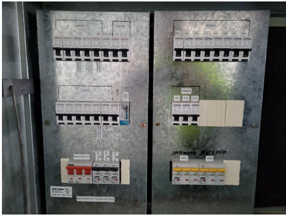
Figure 9-6: Distribution Board in the Rollerama
