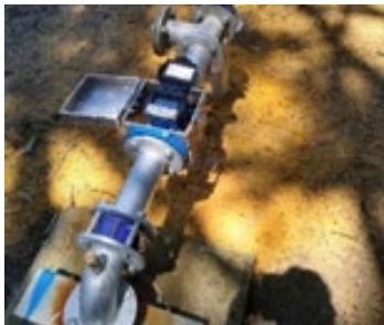
Upgrade of the Bore headworks with a New Octave ultrasonic water meter fitted at the MAR
