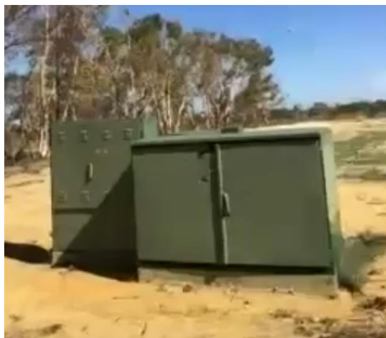
Figure 5-7: Existing, un-used transformer equipment on site and adjacent to landfill
