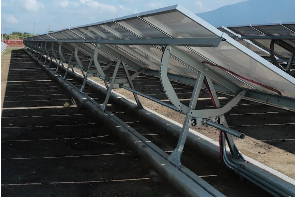
Figure 5-5: Tracking, non-penetrating solar array mounting system from Alion
