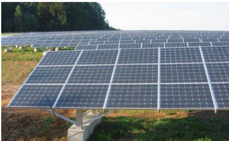
Solar Farm - Pioneer Park
