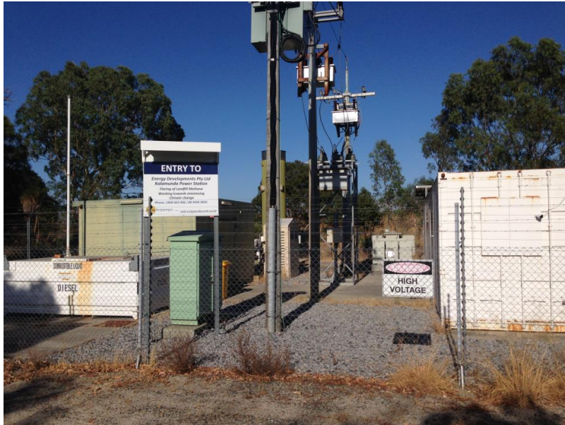
Figure 5-6: Grid connection for existing landfill-gas generator
