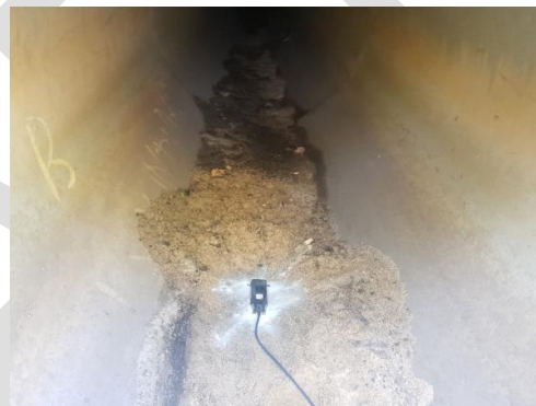
Doppler Sensor installed at Crumpet Creek
