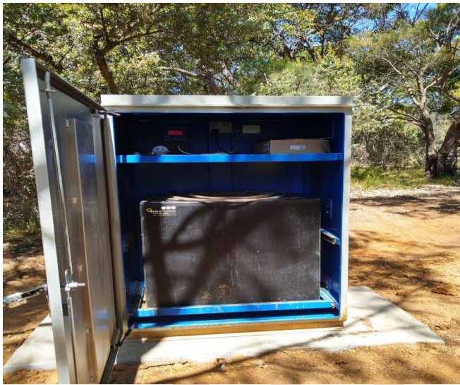
Automated dosing system installed at Ray Owen Reserve
