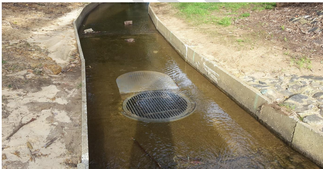
Woodlupine Main Drain stormwater extraction point
